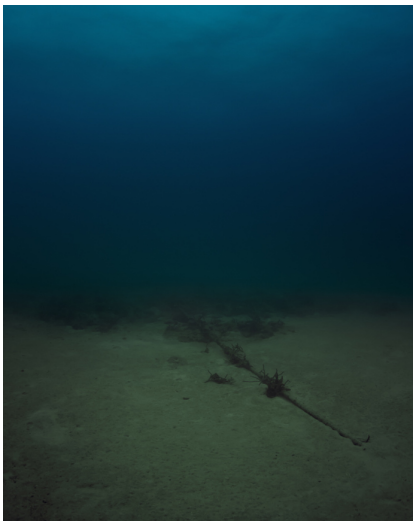
An undersea cable off Miami
